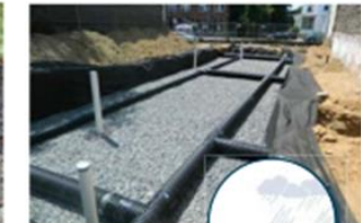
Speichern in Rigolen
